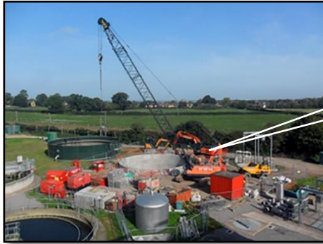
One of the 10m deep settlement tanks that form part of the £3million investment.
